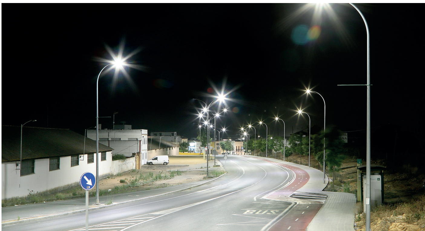
Street lighting 📍 Marinera de Alcor (Sevilla)
